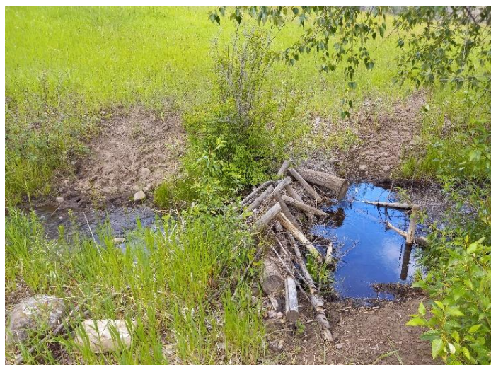
Post-assisted log structures can increase the ability of streams to capture sediment and increase the resilience of riparian areas to wildfire.
