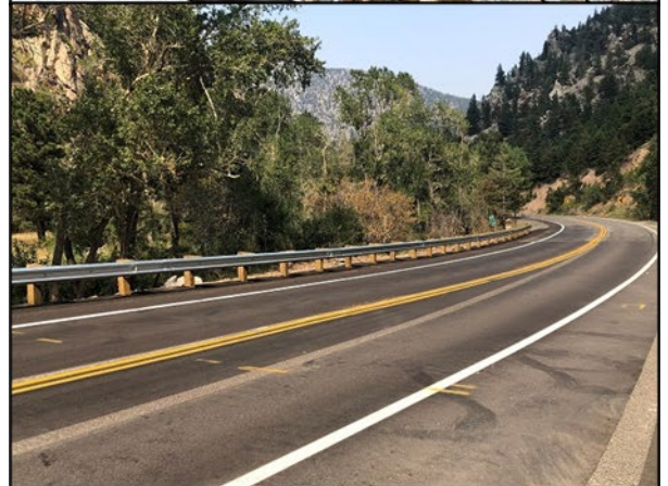
CDOT spent $9.55 million in 2019 and 2020 to make permanent flood repairs along a 12-mile section of CO-72 in response to major flooding in 2013. Photo credits: CDOT.
